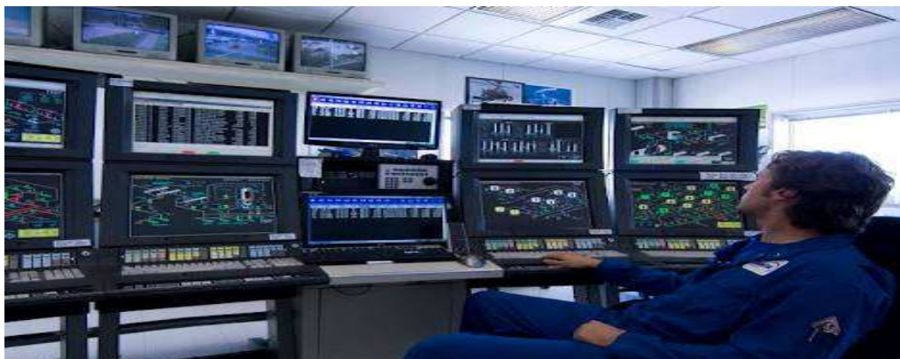
Gambar 4. Ruang Monitoring Operator DCS
